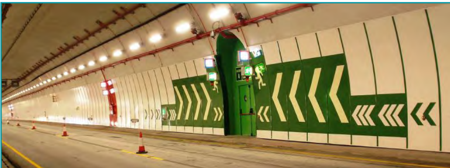
Image 55. Emergency exit (green color) in the tunnel.
